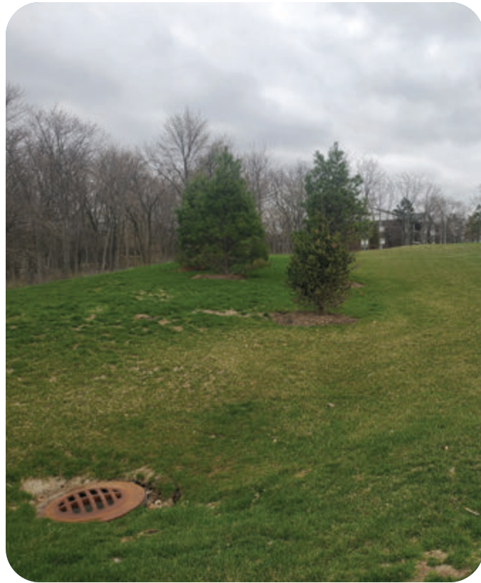
Several inlets on site fail to capture water as it travels from the eastern side of the site down to Crooked Lake.
